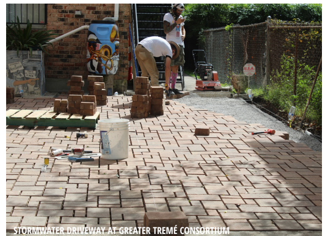
STORMWATER DRIVEWAY AT GREATER TREMÉ CONSORTIUM
